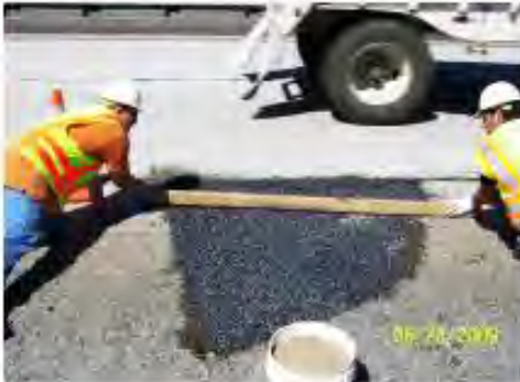
The area is leveled off with a simple 2x4 or straight edge and another pass of Concrete Welder is made to cement the Black Diamond into position.
