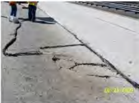
The area featured has sunk 2" to 3" below grade and has significant voids below the surface. Prep is a simple blast of compressed air to remove any loose debris and dirt at the surface.
