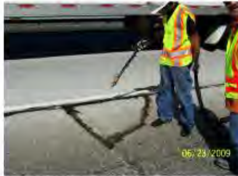
The area, now clean and dry, is flooded with the Low-Viscosity Concrete Welder polymer which flows freely into the voids.
