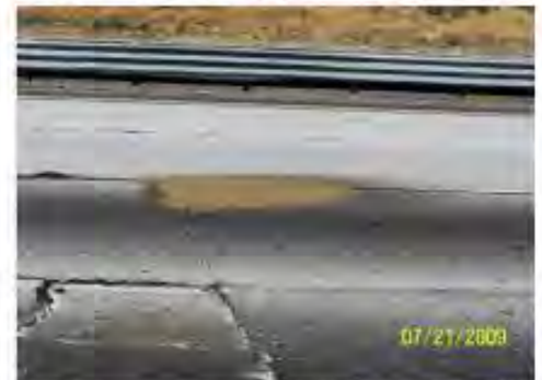
One month later the restored slab is still holding up well while the untreated slab continues to deteriorate.
