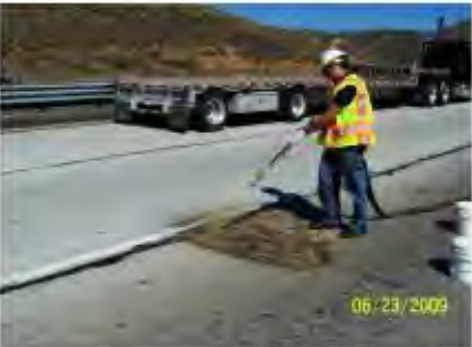
Another pass of Concrete Welder locks the #3 and 3/8" Black Diamond into position.
