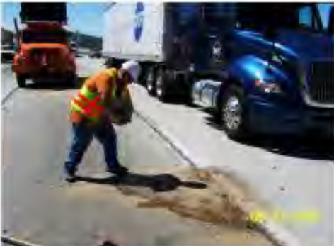
A final pass of #3 coated sand provides a high-traction surface ready for traffic in 10 minutes or less.
