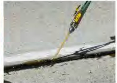
The rapid-setting polymer sets up quickly, allowing for a free flow into the void and then, when gelling, creates a back-fill point.
