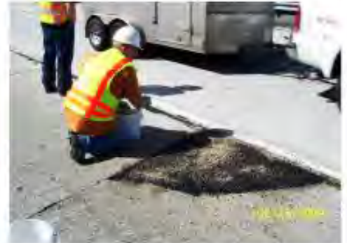
A polymer-coated #3 rounded aggregate is then sprinkled into the base of Black Diamond which provides stability and a good mechanical interlock.
