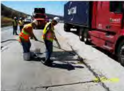
Once sealed and stabilized a 3/8" polymer-coated Basalt known as "Black Diamond" is placed into the depressed area to just below grade.
